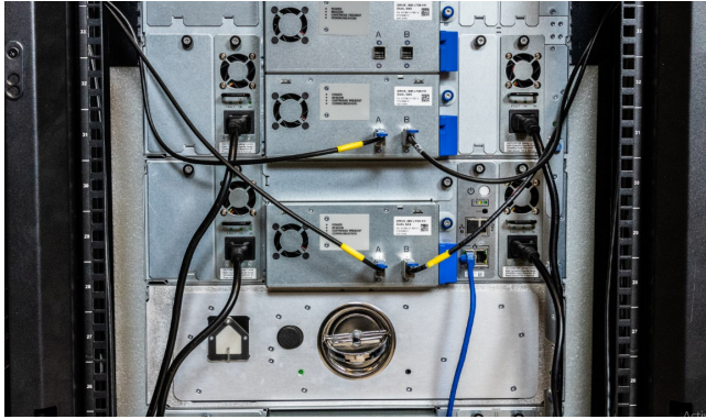
Figure 15: Inspect All Cables and Power Cords
