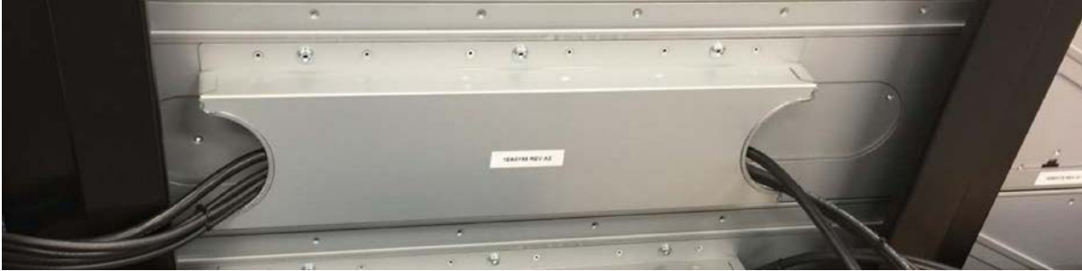
Figure 3-98. Back Rack SAS Cable Channel
