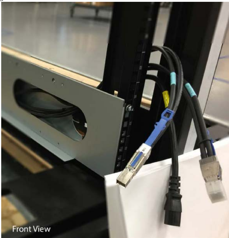
Figure 3-99. SAS Cables and Power Cable Front Vertical Routing
